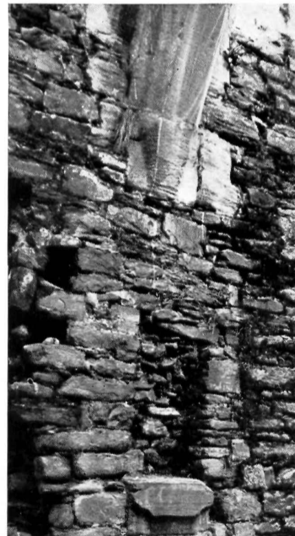
Corbel and slot for roof beam below later arch in Great Hall, S. wall (p. 50ab). Late 13th and mid 14th-century.
