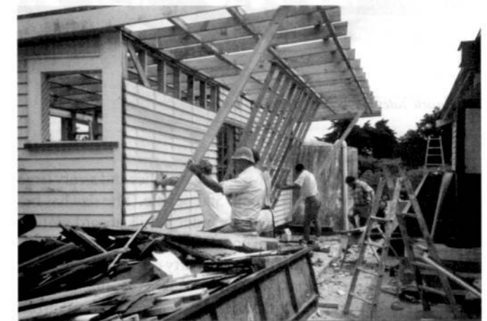
School remodel - the community had enormous input of both money and labour into this project allowing many enhancements to be made. Here the toilet block is being moved.
